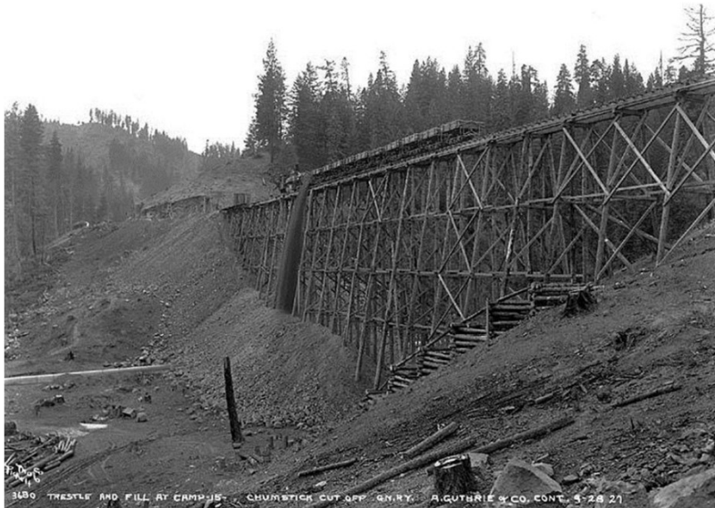
Side-dumping rail cars or wagons from temporary wooden trestles used in construction of large embankments
